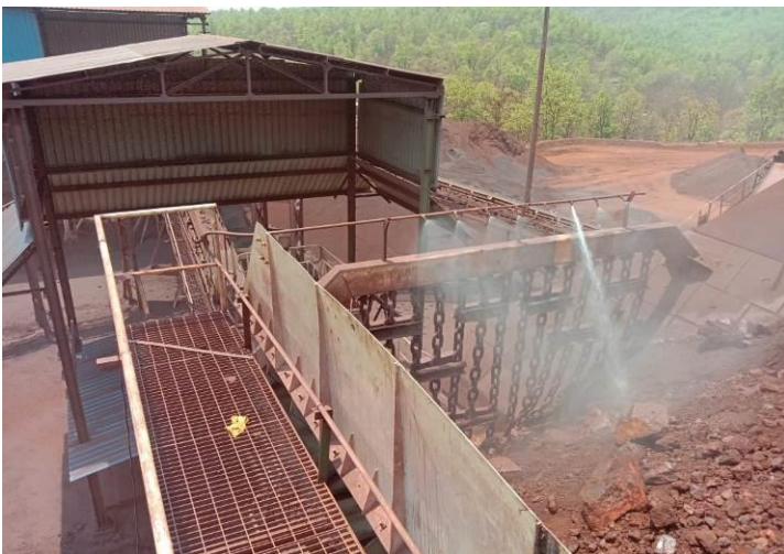
Photo #1D showing dry fog system installation in Crusher & Screen plants
