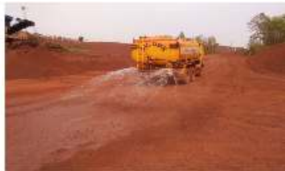
Photo #2B & 4 Showing 20 Kl Water Tanker For Dust Suppression On The Haul Road
